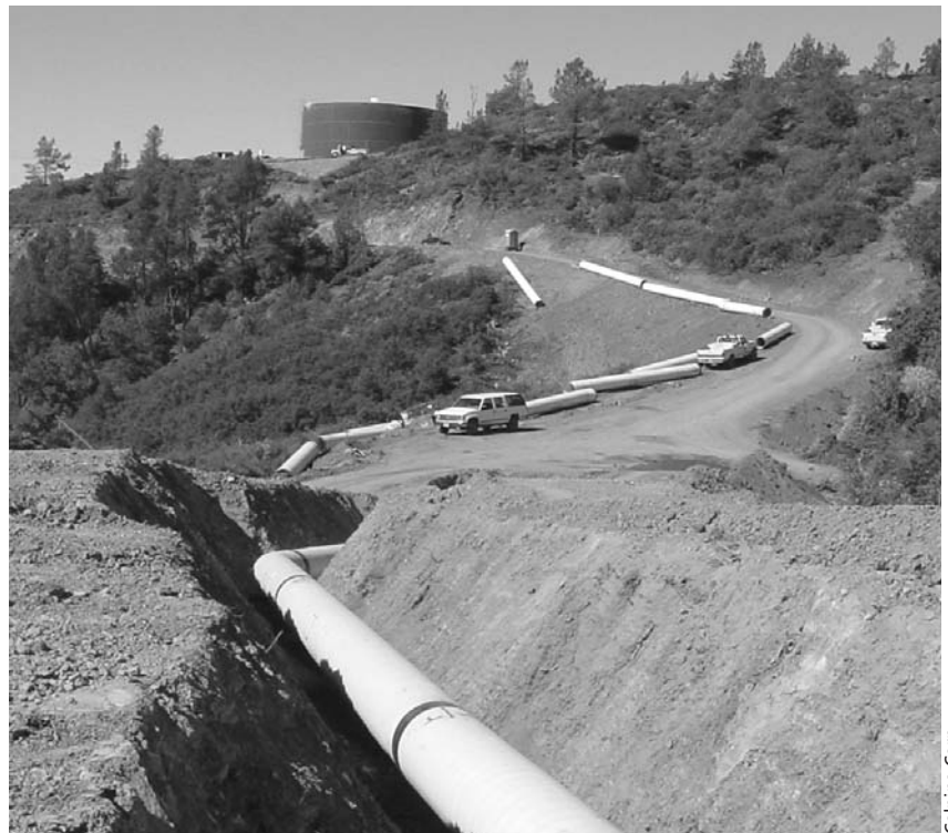
A section of the Santa Rosa Geysers Recharge Project pipeline under construction.
