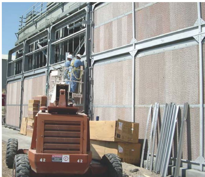
Mammoth-Pacific installed experimental evaporative cooling systems last year, boosting power production as much as 20 percent.
