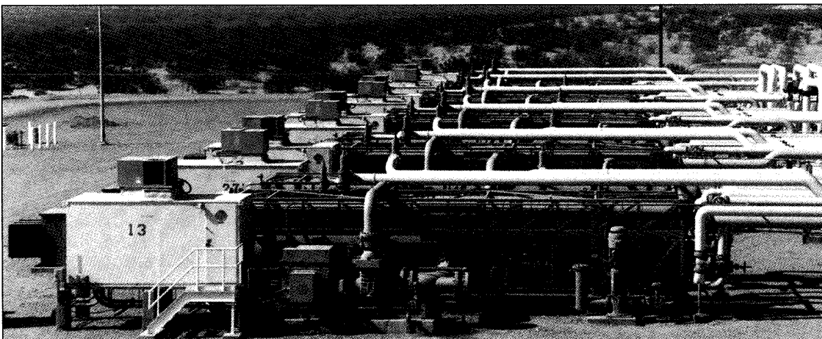
ORMESA II Power Plant comprised of 20 modular Ormat Energy Converters with 20 MW nameplate capacity, synchronized to the IID grid in December 1987.
