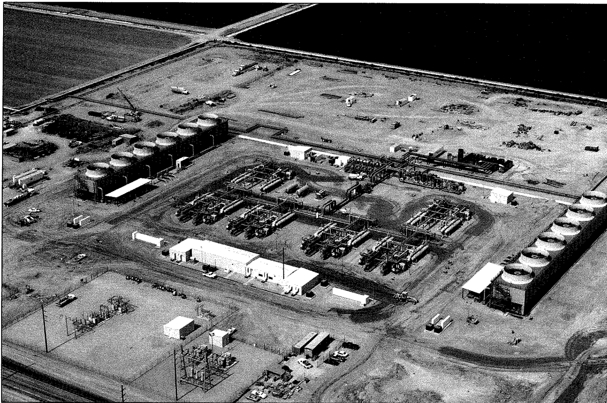
ORMESA II Power Plant comprised of 20 modular Ormat Energy Converters with 20 MW nameplate capacity, synchronized to the IID grid in December 1987.
