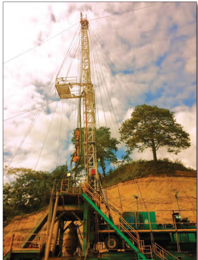
Rig Sky by Steven Fercho . Taken as a storm approaches while drilling Ormat's Platanares, Honduras project. GRC PHOTO CONTEST 2016
