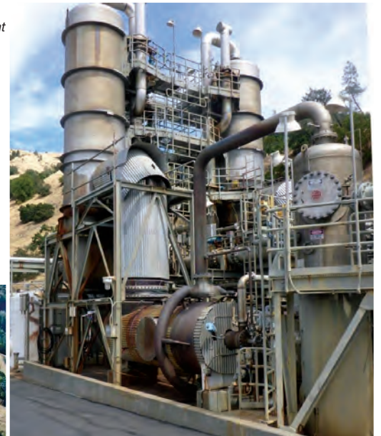
Figure 7: Abatement burner at McCabe Power Plant
