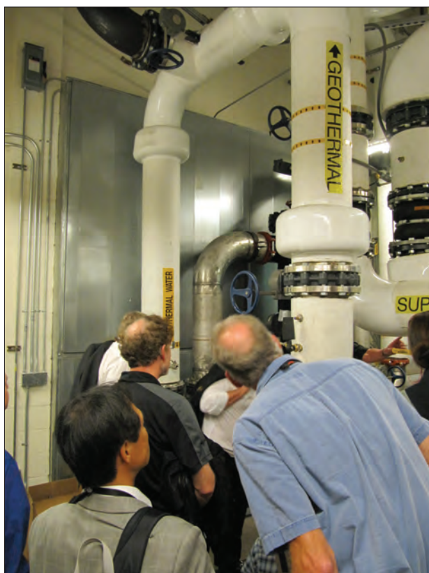
Attendees on a previous tour of the Central Plant facility at the Peppermill observe the use of geothermal waters to provide heat at the resort.
