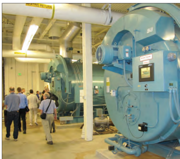
New sources of geothermal heat allowed the Peppermill to retire its Cleaver Brook natural gas boilers in 2009.
