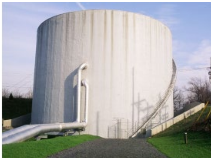
Figure 24: Cornell Chilled Water Storage Tank. Thermal storage tanks like this 4.4 M gallon storage tank on Cornell’s campus allow operators to shift periods in which chilled (or hot) water is generated, thereby shifting the timing of electrical usage for chillers (or heat pumps) used to generate the resource.
