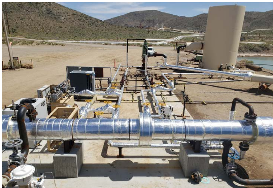
Figure 3: The layout of surface equipment along with wellhead modifications that were required for the demonstration project conducted by GreenFire Energy at Coso, California. The project was funded by the California Energy Commission.
