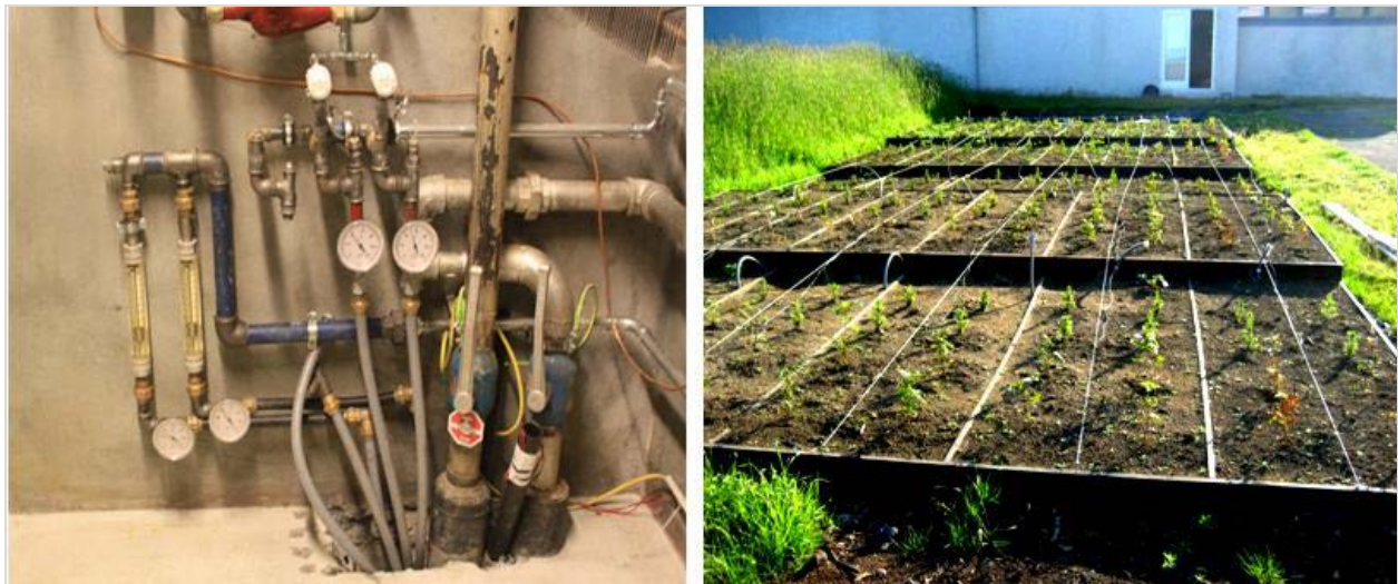
Figure 3: Keilir control system and the gardens
