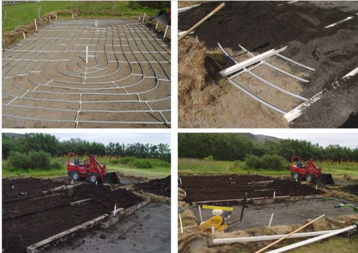
Figure 1: Garden construction process showing the plastic pipe configuration and the over layers
