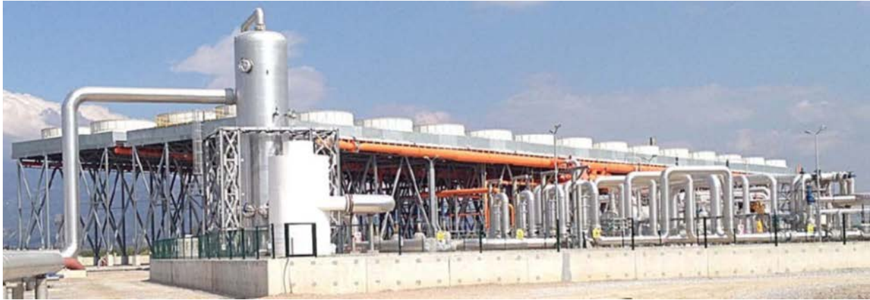
Figure 2: JES-1 power plant, Incirlioiva geothermal project, February 2019.
