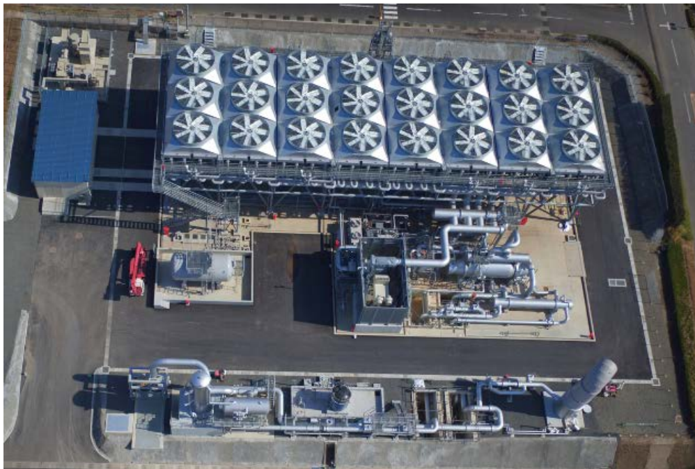
Figure 2: Overview of the Yamagawa Binary Power Station
