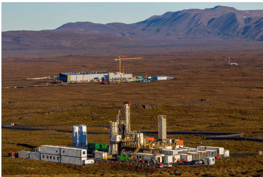
Figure 8: Civil construction well underway; foreground is the drill site for ThG-12, autumn 2016.
