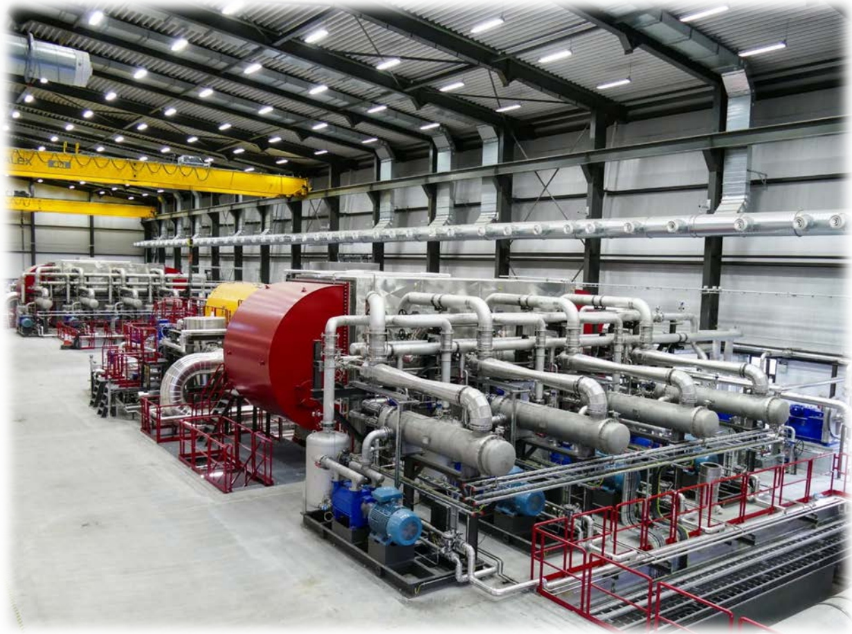
Figure 3: Turbine/generator units. Unit 2 in the foreground and unit 1 in the background.
