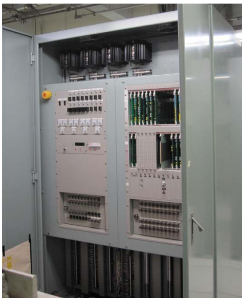
Figure 2: Original MHI Electro Hydraulic Control System Cabinet
