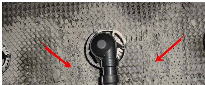
Figure 5. Areas of heavy sulfur fouling beneath spray nozzles result in uneven water distribution through the cooling tower fill, and damage to the fill (red arrows).
