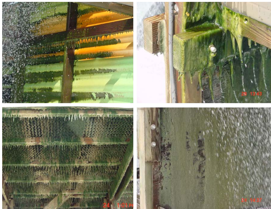
Figure 3. Algal and microbial fouling was evident throughout Unit #12 cooling tower.
