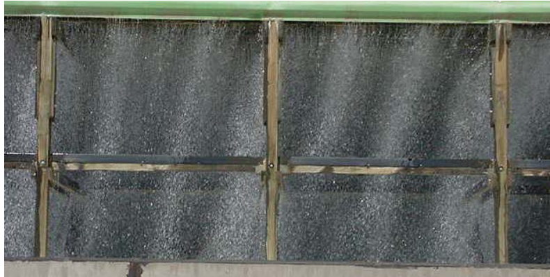
Figure 6. Channeled flow due to uneven water distribution beneath sulfur-fouled spray nozzles.
