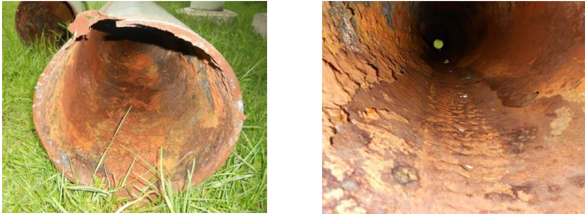
Figure 3: Corrosion of steel pipes at Wanyang Windu due to chemicals in condensate
