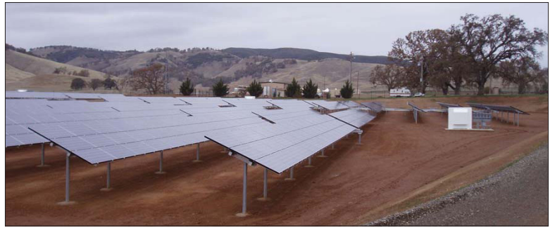
Figure 17. PV system with the pump house (in back) for the Southeast Geysers Effluent Pipeline (Enezy and Rudisill, 2009).
