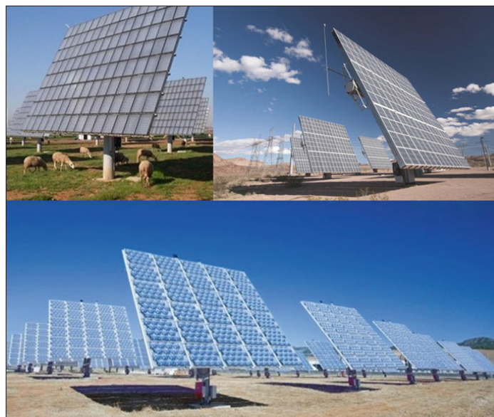
Figure 2. PV panels (Ritcher et al, 2012).
