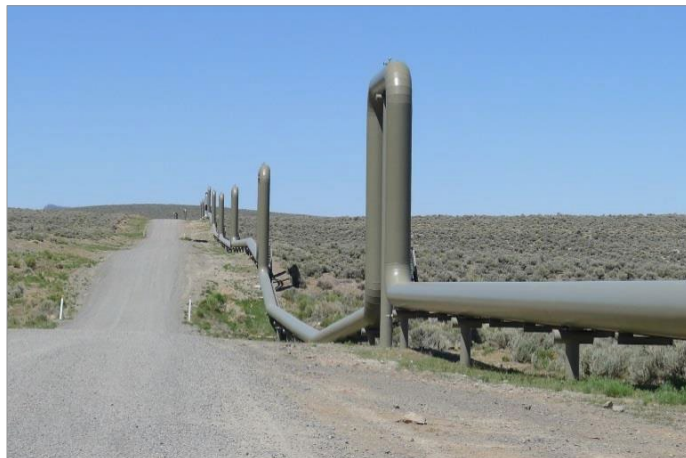
Figure 11. Geothermal pipeline expansion loops at the McGinness Hills project.
