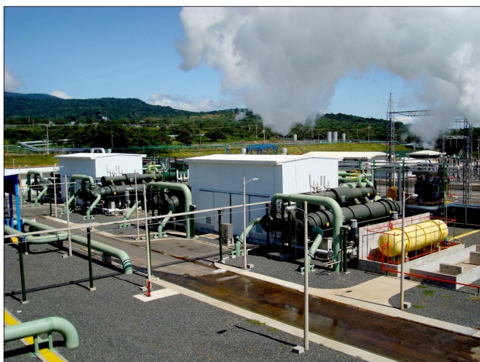
Figure 14. Power houses for Unit 1 (left) and Unit 2 (center). Condensers and recuperators are the dark-colored horizontal vessels adjacent to the buildings; the N-pentane holding tank is the yellow horizontal vessel at the right. Photo by P. Moya.
