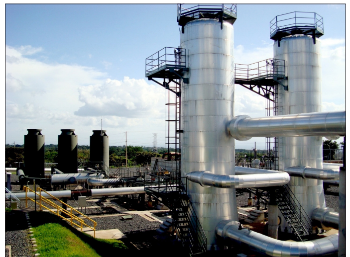
Figure 11. Separator station; twin cyclone separators in foreground and bank of silencers in background. Photo by P. Moya.
