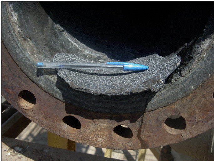
Figure 1. Silica scaling in the water discharge of a primary steam separator.
