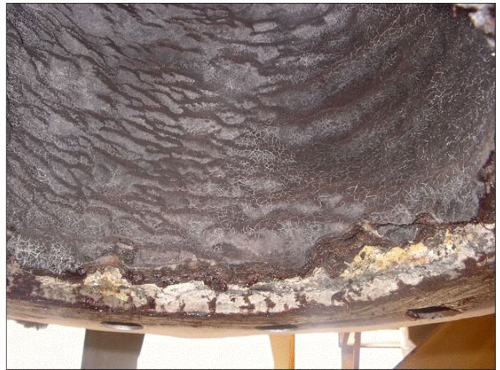
Figure 2. Silica scaling in the water discharge of a secondary steam separator.
