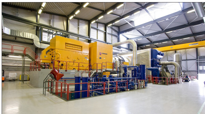
Figure 4. Turbine generator unit no. 1.
