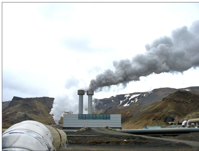
Figure 3. Steam valve house for units 5 & 6, at steam blow out.
