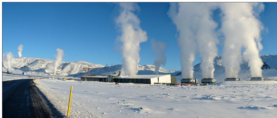
Figure 1. The Hellisheiði power plant.
