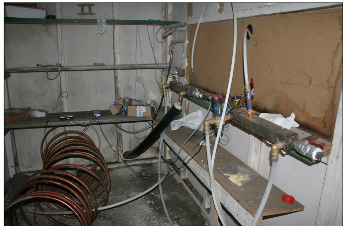
Figure 6. Setup of the testing and datalogger equipment inside the shed at the Keldunes location.
