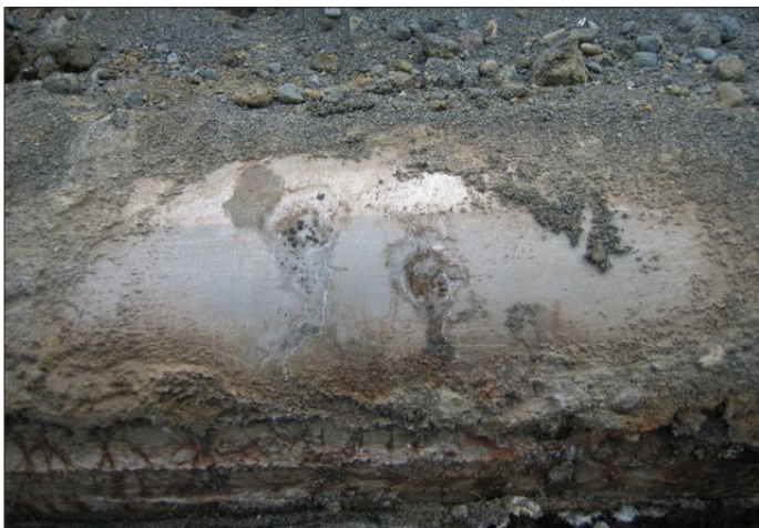
Figure 7. Outward corrosion of the steel pipes.
