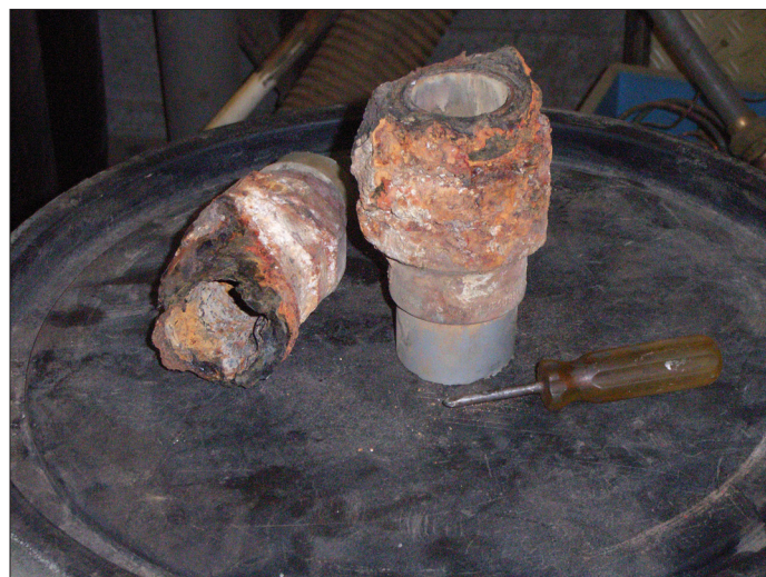
Figure 9. Corroded joints from the distribution system in the heating system in Öxarfjörður.
