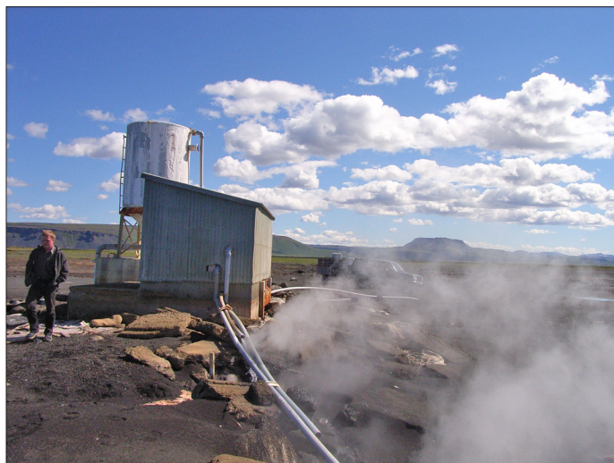
Figure 5. The well head of the production well in Skógálón. The polybutylene pipes are seen in the foreground. A steam separator used in the years 2005-2006 is seen in the background.
