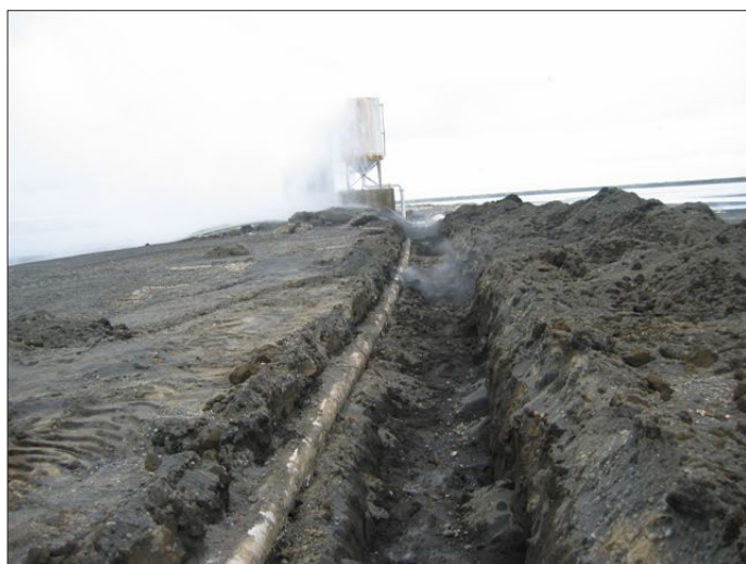
Figure 6. A View towards north to the well, showing the steel distribution pipe being dug up for replacement in 2006.
