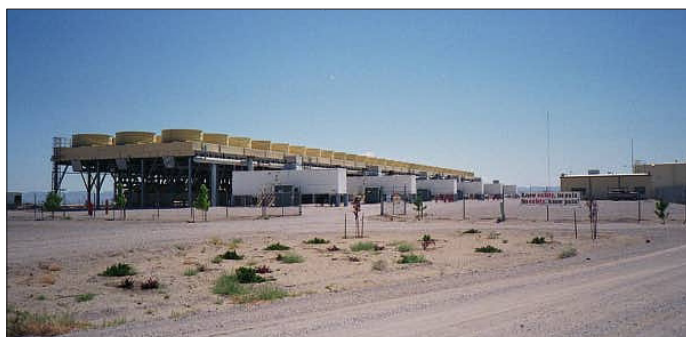
Figure 2. A typical small fan air-cooled condenser on a geothermal power plant.
