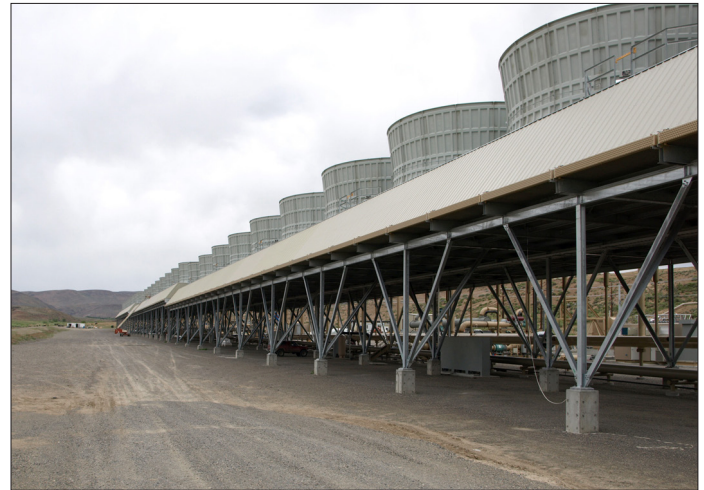
Figure 5-1. Site Photo of the New Design Air Cooled Condenser.
