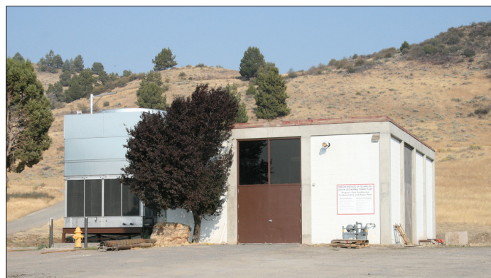
Figure 5. The building on the OIT campus housing the 280 kW power plant, with the wet cooling tower on the left.
