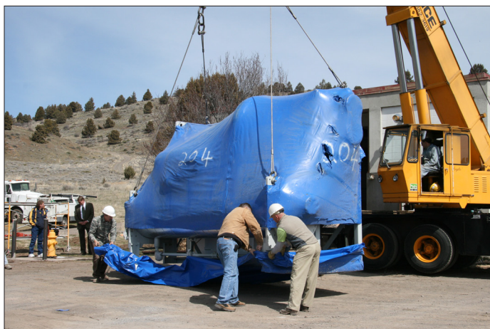
Figure 2. Delivery of the UTC Pure Cycle© 280 kW binary power plant.
