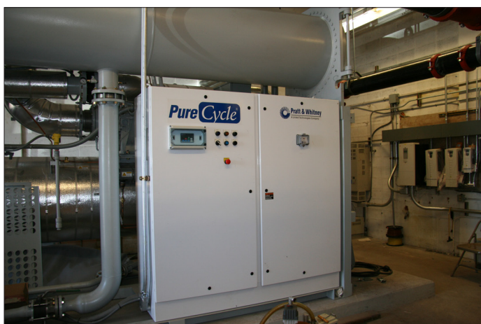
Figure 4. The control panel for the 280 kW binary power plant.
