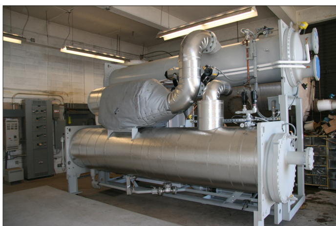
Figure 3. The 280 kW binary power plant with the turbine-generator set (covered). The condenser shell-and-tube heat exchanger is on top and the evaporator on the bottom.
