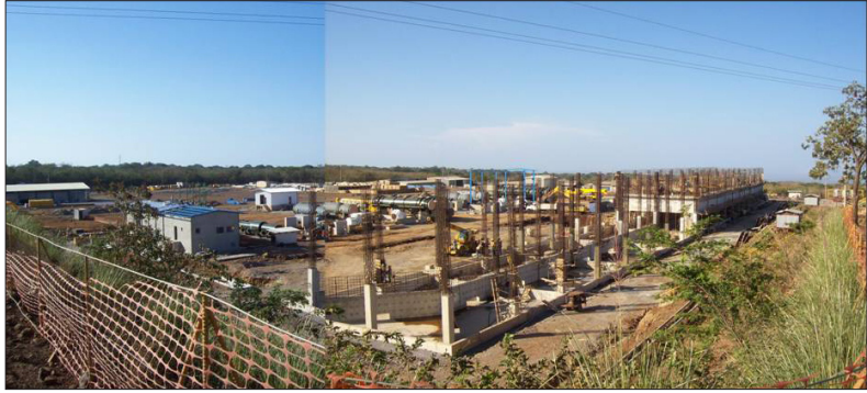
Figure 3. Recent photo mosaic of the advance of construction the Pailas Geothermal Plant (March 3, 2010).
