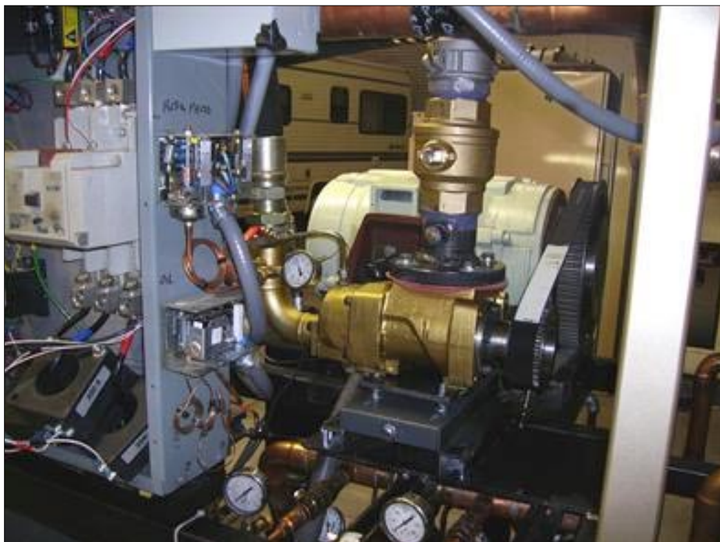
Figure 9. ORC Demonstration Unit.
