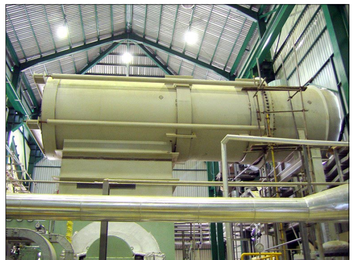
Figure 3. Photo of Turbine unit.
