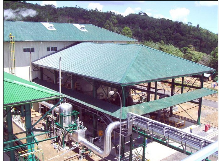
Figure 5. Photo of Power station.
