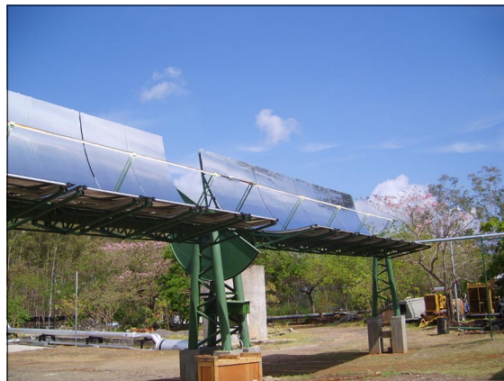
Photo 1. PTC and AH-6 geothermal well facilities.
