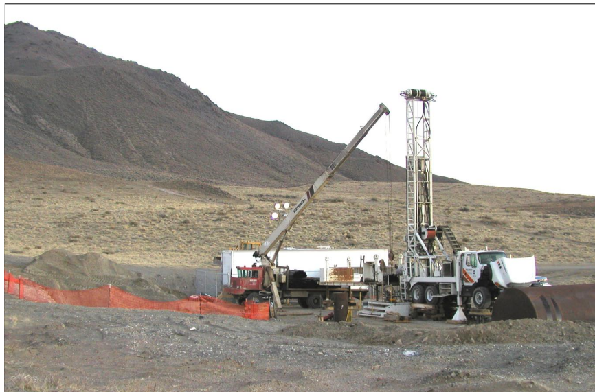
Figure 5. Drilling of the Blue Mountain No. 2 well by Nevada Geothermal Power, Inc. in 2004. Measured fluid temperatures exceeded 160^{\circ}\text{C} and geothermometer temperatures are >200^{\circ}\text{C} (Niggemann et al., 2006).
