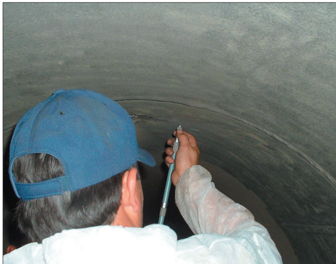
Picture 2. Steel cleaned with low corrosion attack.
