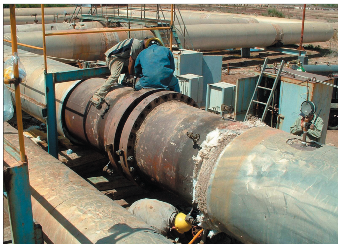
Picture 3. New pressure arrangement with four taps.
