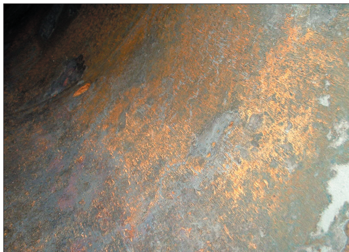
Picture 4. Inside pipeline intermediate pressure before cleaning job, with no evidence of corrosion problems.
