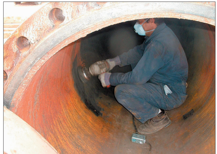
Picture 1. Internal aspect of the pipeline before cleaning job. High pressure pipeline.
