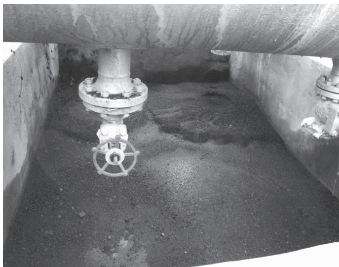
Figure 12. Debris found at the MST drain box.
