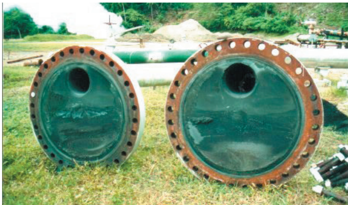
Figure 8. Modified solid trap outlet flanges.
