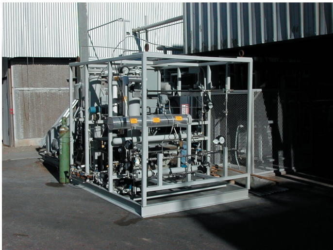
Figure 1. Skid-mounted prototype system installed in host site plant.
