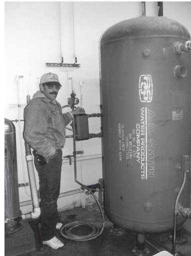
Figure 5. Sand filter in the Aquatic Center.
