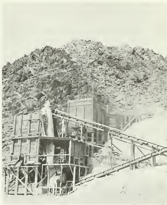
Photo 7. Mill, Lakeview Quartzite deposit: Quarry-run rock is crushed and sized with jaw crushers and a trommel screen to approximately minus 2 inches, plus ½ inch. The fines, which contain most of the impurities, are discarded.
