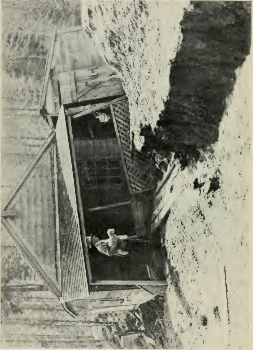
FIGURE 14. O'Rourke 1950 slump. House was damaged by movement of differential blocks of the slump.
