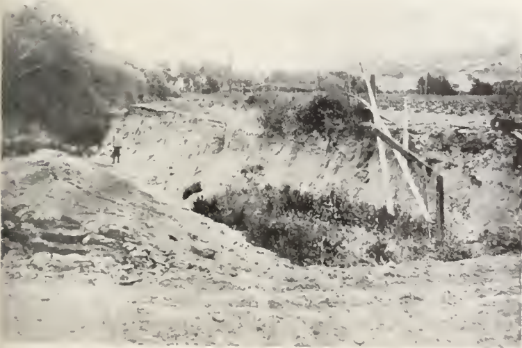
FIG. 17. Disrupted roadbed near Spreckels, Salinas Valley, caused by lurching in deep alluvial fill. San Andreas fault passes through on the other side of the Gabilan Range in the vicinity of San Juan Bautista, many miles to the east. Some of the secondary results caused by shocks produced at times of major faulting often are more spectacular than direct dislocations in the fault zone itself. Photo from the J. C. Branner collection, courtesy Stanford University.
