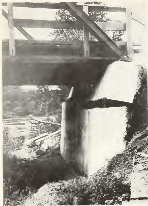
FIG. 21. Bridge abutment at Chittenden on the Pájaro River, Santa Cruz County, disrupted by earth movement connected with the earthquake of 1906. Photo from J. C. Branner collection, courtesy Stanford University.
