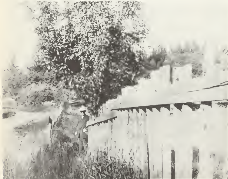
FIG. 7. Offset fence near Wright Station, Santa Cruz Mountains—a typical disruption of linear features that happened to cut across the San Andreas fault. Fault movement was predominantly horizontal but many complexly operating forces were active within the fault zone. Photo from J. C. Brunner collection, courtesy Stanford University.
