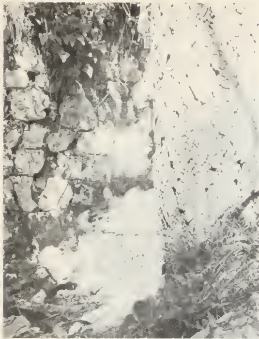
FIG. 5. Photograph taken inside kiln 3, showing small Douglas fir growing in kiln. Stone mason work of inner casing has been carefully done. Photo by J. Quast.
