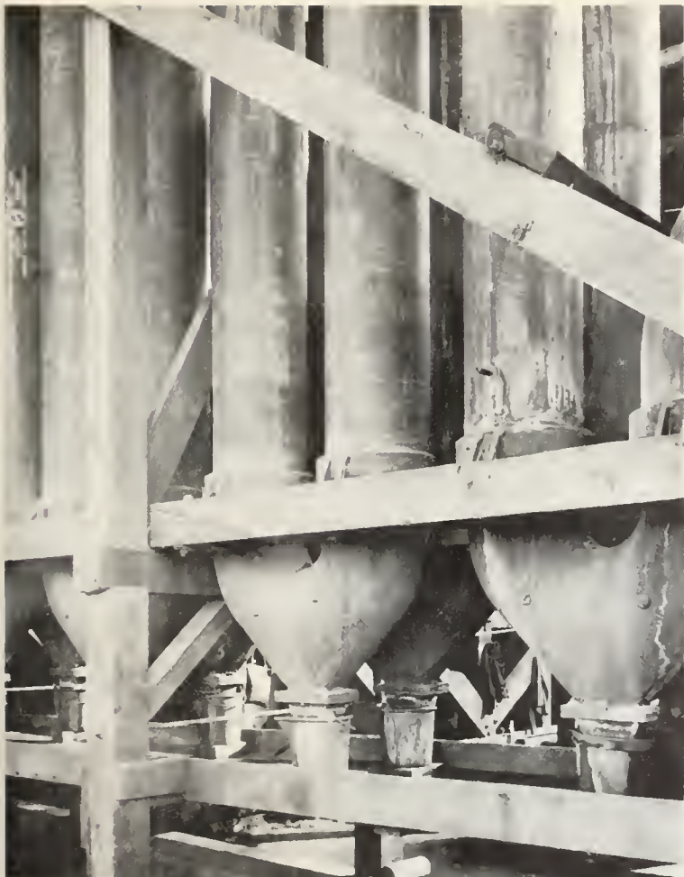
FIG. 3. Close-up of condenser tubes in a typical quicksilver-refining mill, New Idria, San Benito County. Photo courtesy Pacific Gas and Electric Company.
