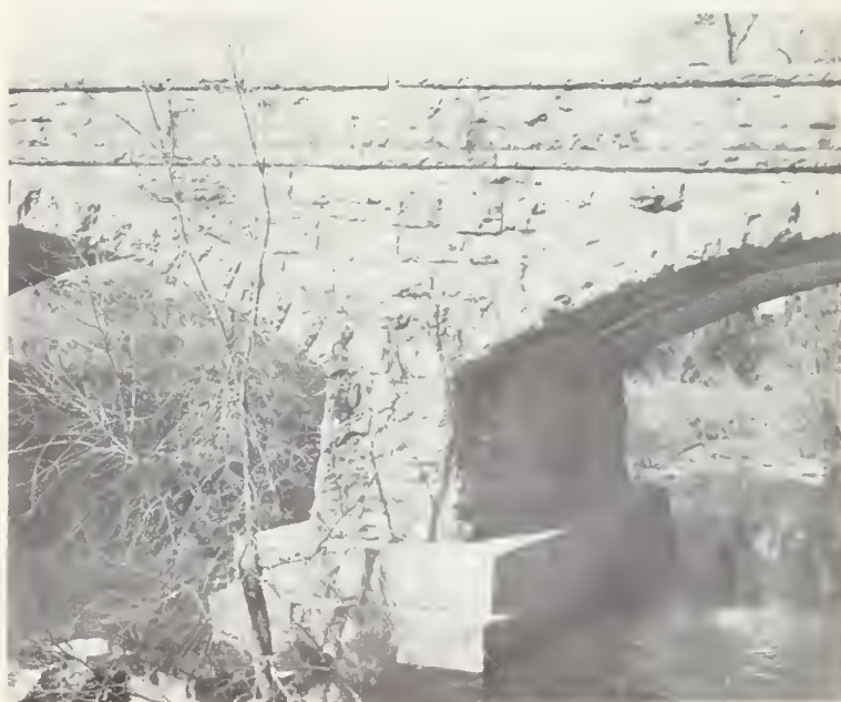
FIG. 5. Napa Creek Bridge, northeast of Zinfandel, Napa County. Constructed in 1913 of perlite rock, dacite, and rhyolite.
