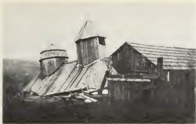
FIG. 11. The Greek Orthodox Church at Fort Ross as it appeared right after the earthquake of April 18, 1906. Photo from J. C. Branner collection, courtesy Stanford University.
