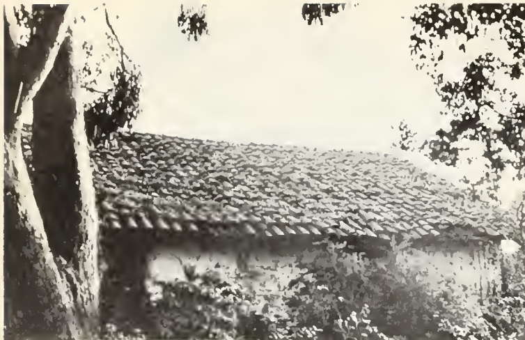
FIG. 5. José de Jesus Vallejo adobe on grounds of California Nursery Company at Niles. Adobe was built about 1850. Photo by Mary Rae Hill.
