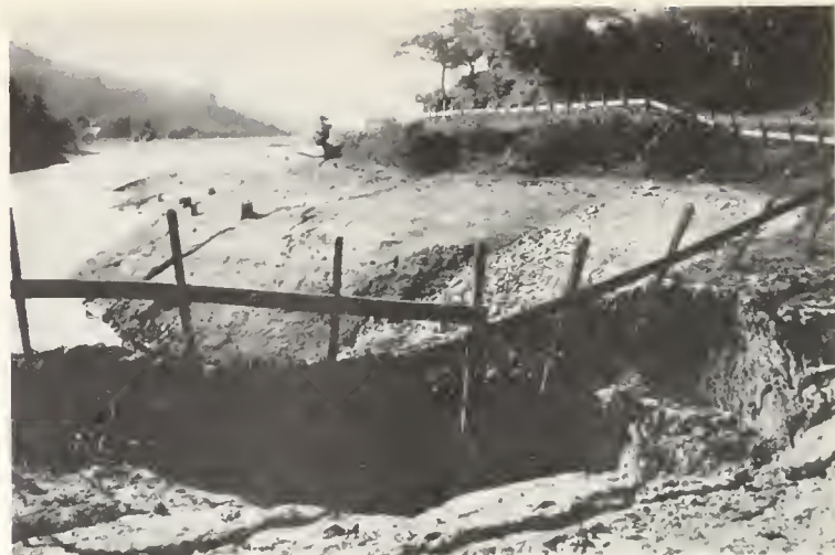
FIG. 12. Reservoir south of Saratoga damaged and partly drained as a result of the San Andreas fault movement of 1906. Photo first published in Carnegie Inst. Wash. Pub. 37, vol. 1, pt. 1, pl. 64A.
