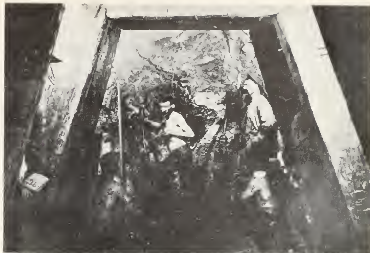
FIG. 6. A working face in the New Almaden Mines showing detail of the massive timbering used to support the ceiling and walls. Note the large rectangular hand-wrought spikes in one of the timbers on the right. Photo from the Bulmore-Winn collection, courtesy Jimmie Schneider, San Jose.
