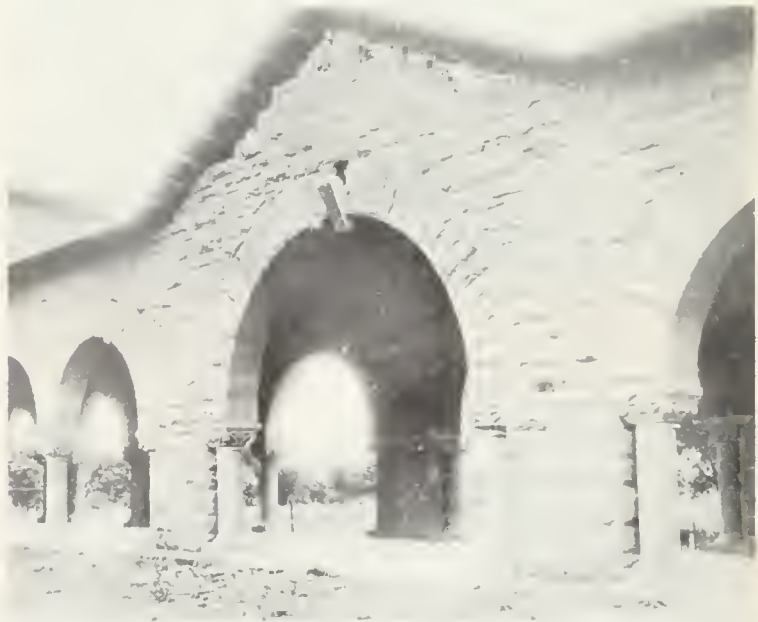
FIG. 10. Part of the arcade at Stanford University, showing displaced keystone in the middle arch, a result of the earthquake of 1906. Photo from the J. C. Branner collection, courtesy Stanford University.
