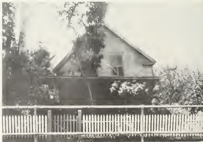
FIG. 4. Frame house at Olema, Marin County, knocked from its foundations during the 1906 earthquake. Wooden frame buildings usually withstand severe earthquakes if bolted to adequate foundations. Photo from J. C. Branner collection, courtesy Stanford University.
