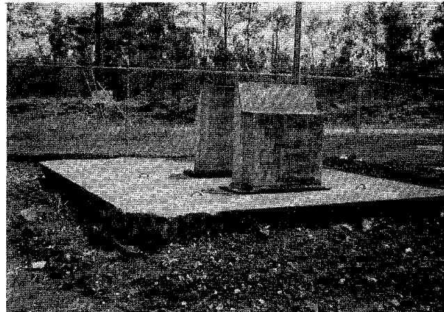
Lid to the concrete bunker built around well HGP-A.
