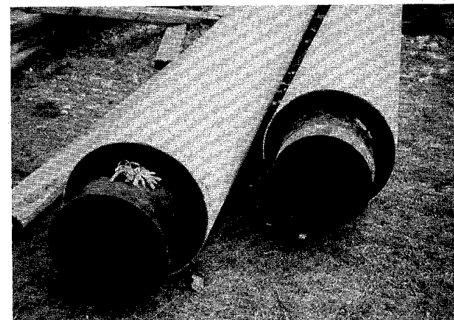
FRP (fiberglass reinforced plastic) insulated geothermal water distribution pipes, before installation in the Oregon Institute of Technology (OIT) system.
