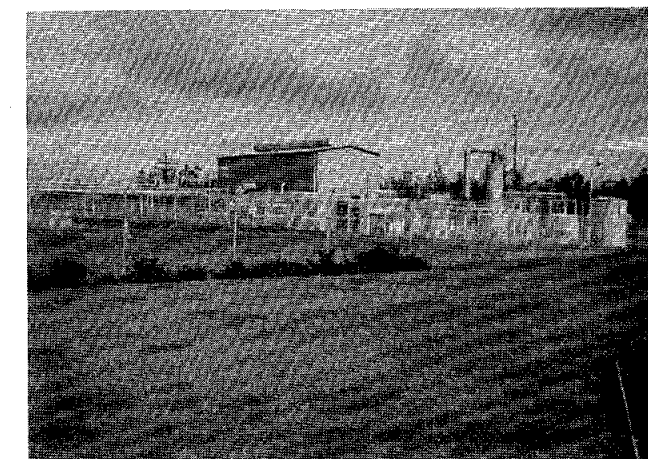
The Hawaii Geothermal Plant. The 3 megawatt plant is constructed at the well site. The turbine and generator are modular units that can be lifted with a bridge crane. Whenever volcanic eruptions threaten, these elements can be placed on a trailer and hauled away. Photos by Susan F. Hodgson.
